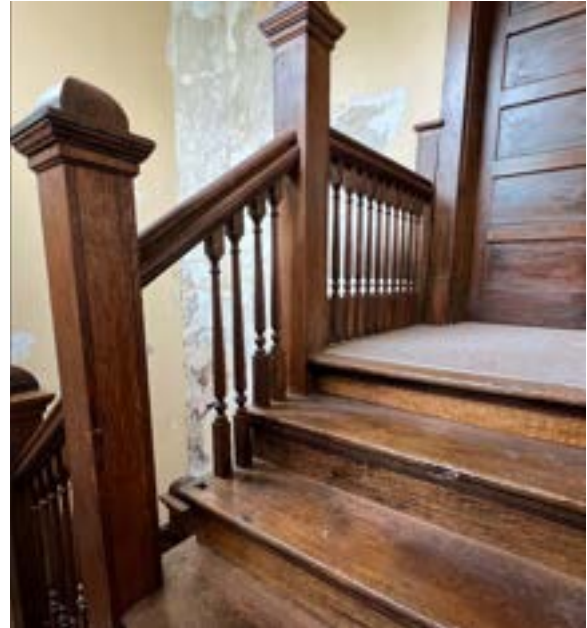
Figure 2.229. Missing baluster on upper section of eastern stair. Photo by author.
