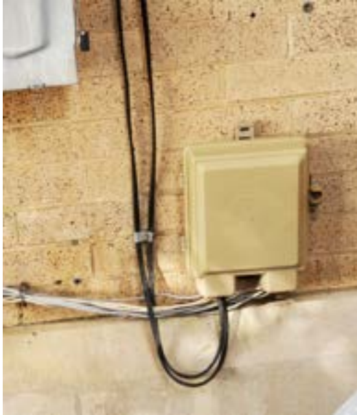
Fig. 2. 297 Landline telephone drop on southeast corner of building. Photo by author.
