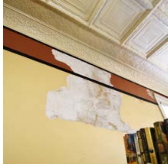
Figure 2.205. Damage along the side of first floor interior wall. Photo by author.
