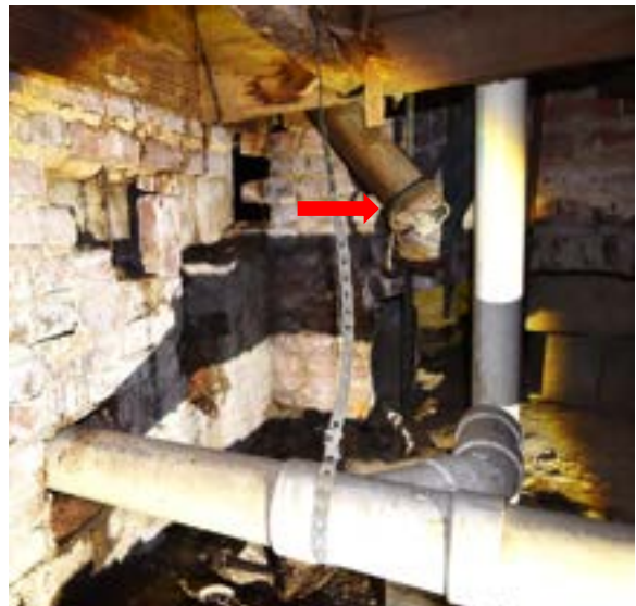
Figure 2.306. Cast iron waste lines (red arrow) replaced with PVC. Photo by author.
