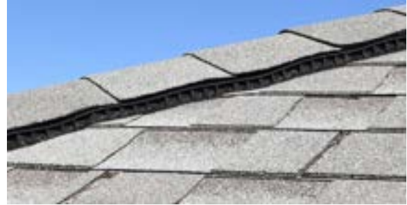
Figure 2.53. Ridge vents line the crest of asphalt roof. Note that missing ridge vents will be identified in a later section of this report. Photo by author.
