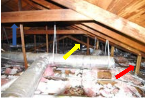
Figure 2.50. Rake cut vertical studs support rafters (red arrow). Large angle braces catch end of north/south ridge board (yellow). Collar ties (blue) run approximately every third bay. Photo by author.
