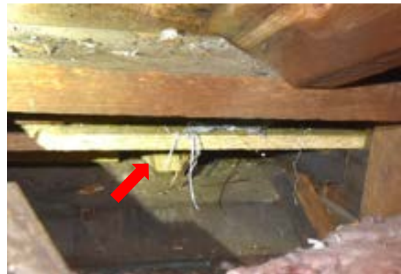
Figure 2.62. Evidence of repairs to box gutter in northeast corner. Note the pressure treated lumber visible (highlighted with red arrow). Photo by author.
