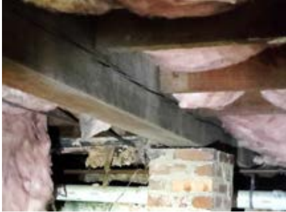
Figure 1.69. Main floor system carrying beams are 6" x 8" single timbers measuring 26' in length. A mammoth piece of wood representative of a past era. Photo by author.
