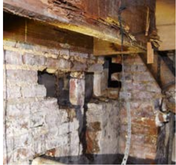
Figure 2.17. Extensive material failure to eastern stairway wall at junction with interior masonry wall. Note vertical bricks providing support. Photo by author.
