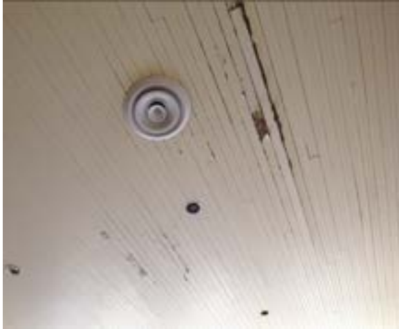
Figure 2.269. Damaged beadboard in 2nd floor main room (east). Photo by author.
