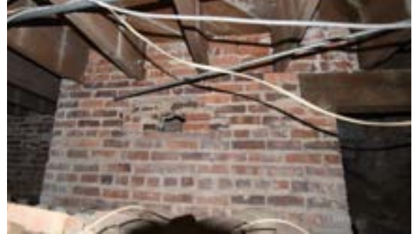
Figure 2.10. Large hollow box piers supporting the building's front entry. Photo by author.
