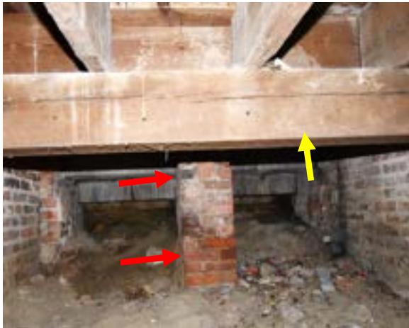
Figure 2.190. The settling of the masonry pier and the supporting wood timber (yellow arrow) may have contributed to cracks in the floor above. Photo by author.
