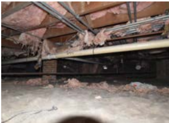
Figure 2.9. Good clearance in crawlspace (42") but access is limited by small foundation windows. Photo by author.
