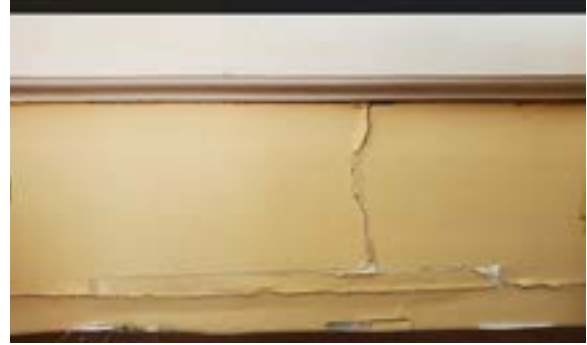
Figure 2.215. Possible water damage on southwest wall in modern addition. Photo by author.
