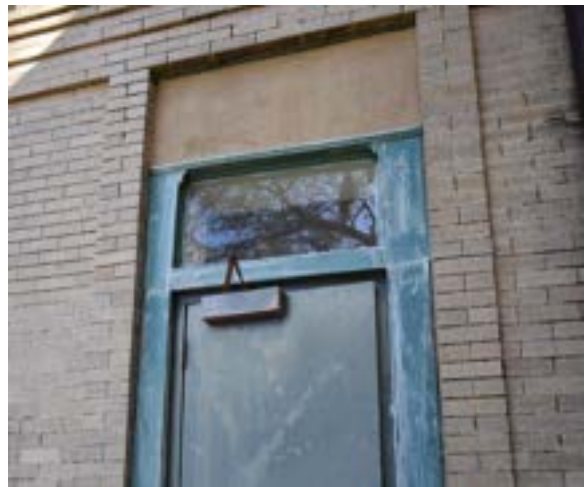
Figure 2.164. Exterior fire exit door. Note EIFS cladding above doorway. Photo by author.
