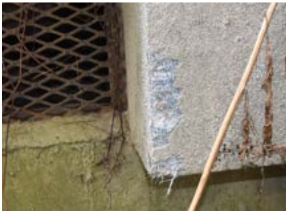
Figure 2.111. All the addition's exterior wall features, like the water table pictured above, are constructed with EIFS. Photo by author.
