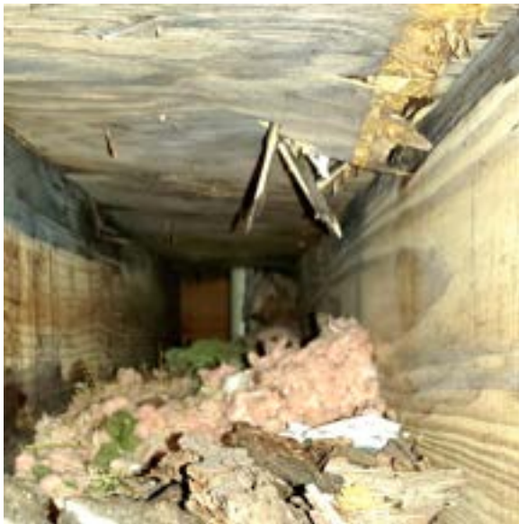
Figure 2.45. Failing floor and organic growth beneath first floor restroom (south). Photo by author.
