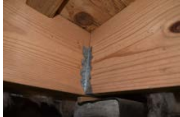
Figure 2.42. Joists attached to carrying beam with Simpson type hangers. Photo by author.
