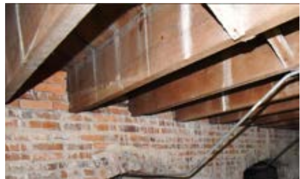
Figure 1.68. The floor system is comprised of 2"x12" (actual) southern yellow pine joists, some measuring 21' in length. Photo by author.
