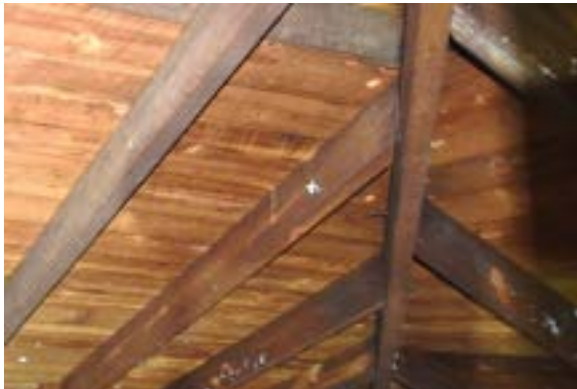
Figure 2.60. Roof framing is sound, and decking is well seated on rafters. Photo by author.
