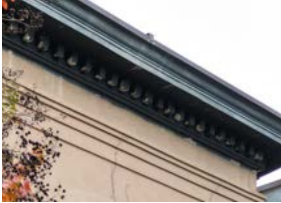
Figure 2.66. The gutter/cornice on the addition is a combination of copper lined gutters and polyurethane molding. Photo by author.
