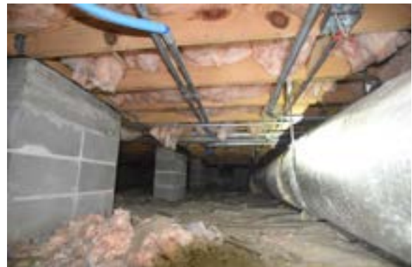
Figure 2.26. Tight access (approx. 32") below the modern addition. Photo by author.
