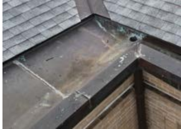
Figure 2.57. Welded seam copper lining in the box gutter troughs. Photo by author.
