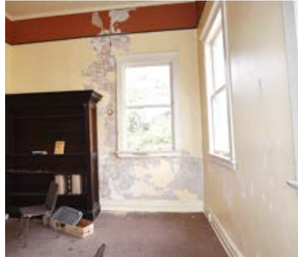
Figure 2.195. Plaster finish is historic, but several sections will require repair and restoration. Photo by author.
