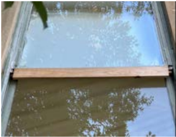
Figure 2.149. Evidence of prior repairs to hold glass in place. Photo by author.
