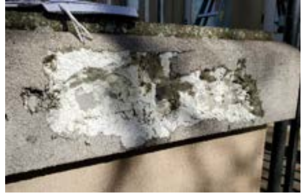
Figure 2.112. Damaged EIFS cladding on ADA ramp pier. Photo by author.
