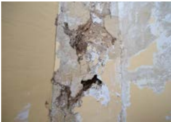
Figure 2.208. Large organic growth in eastern stairwell. Photo by author.
