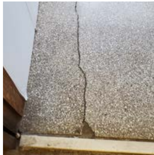
Figure 2.189. Significant crack in main entry terrazzo floor. Photo by author.
