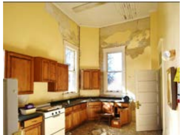
Figure 2.206. Extensive water damage in kitchen on 2nd floor. Photo by author.
