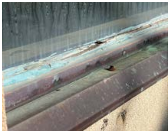
Figure 2.147. Clouded glass and decayed glazing noted on several windows in Addition. Photo by author.
