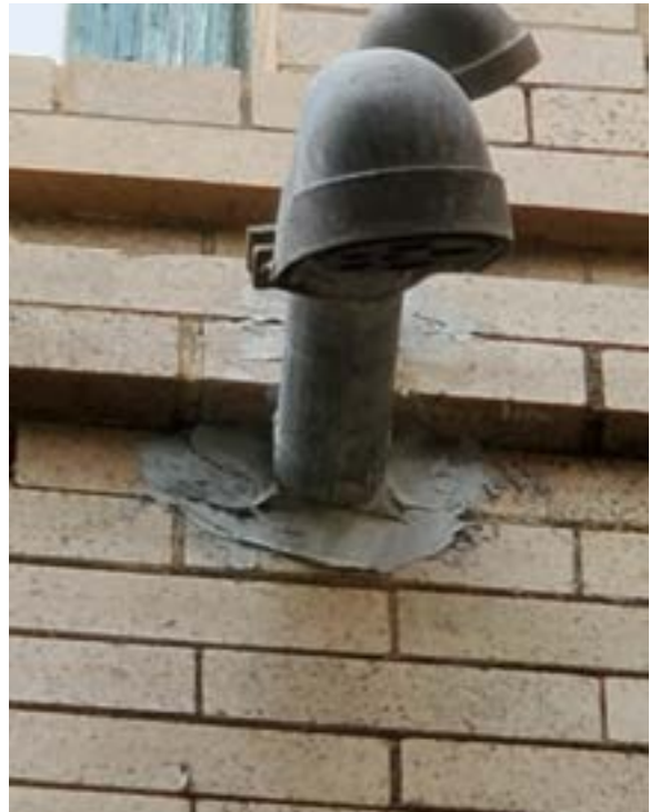
Figure 2.292. Abandoned service hood on building north exterior. Photo by author.
