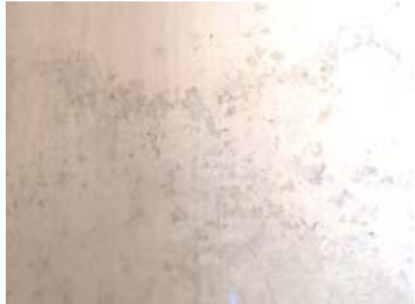
Figure 2.209. Mold growth on walls visible throughout building. Photo by author.
