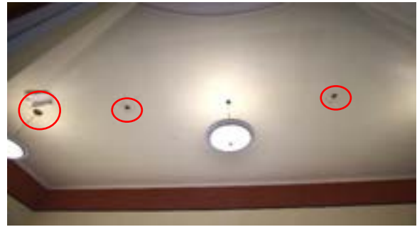
Figure 2.271. Ceiling in modern addition shows evidence of water damage in several places. Photo by author.
