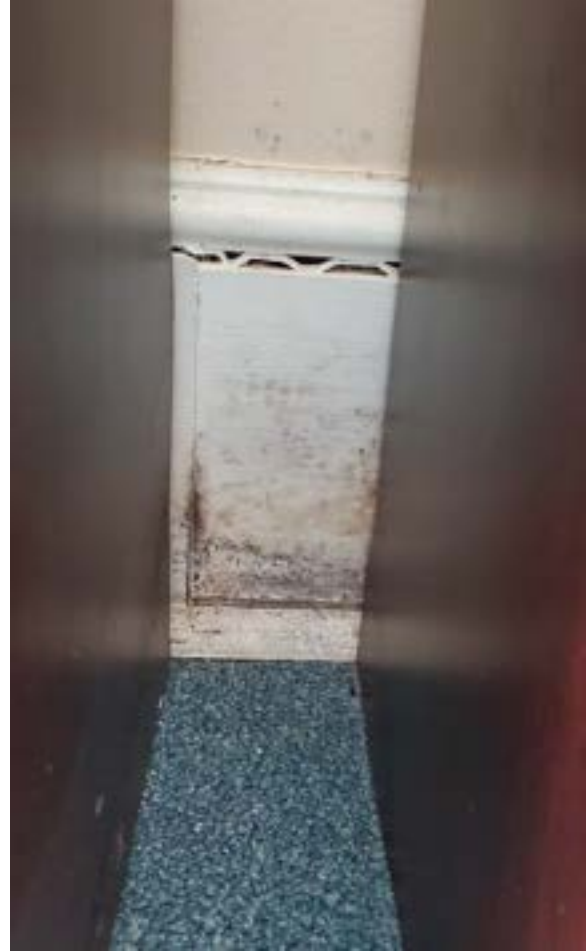
Figure 2.109. Evidence of water penetration and decay on interior baseboard in the addition's northwest corner (partially obscured by bookshelf). Photo by author.
