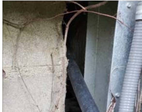
Figure 2.29. The addition's foundation wall was altered (southside) after construction for mechanical pass-through. Structural integrity may be compromised in this section. Photo by author.
