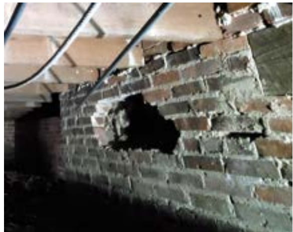
Figure 2.22. Unexplained punctures to hollow box foundations beneath main entry. Photo by author.
