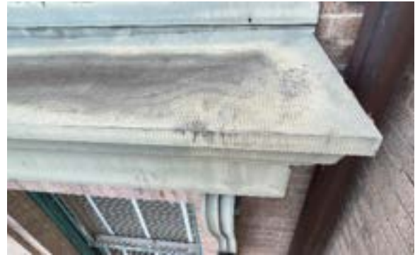
Figure 2.153. Hood H04 shows signs of chronic water pooling. Photo by author.
