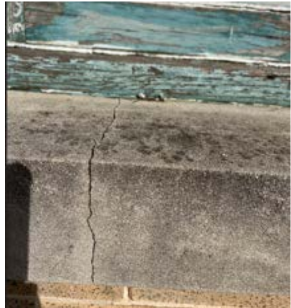
Figure 2.142. Window #112 has a broken belt course sill. Photo by author.
