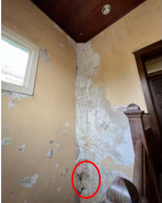
Figure 2.207. Extensive damage in eastern stairwell. Photo by author.
