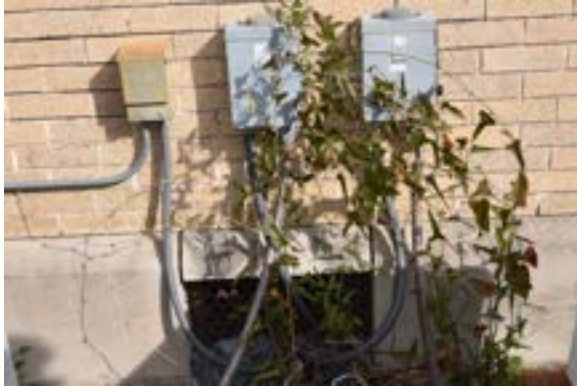
Figure 2.8. Three foundation openings are used for utility/mechanical lines. Photo by author.
