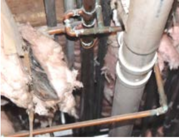
Figure 2.307. Water supply lines are copper. Photo by author.
