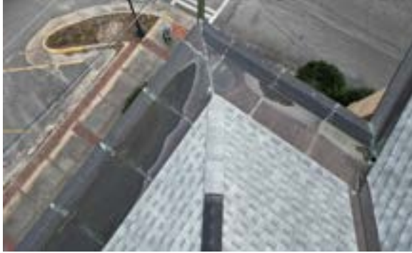
Figure 2.81. Northeast corner box gutter with some water pooling. Photo by author.
