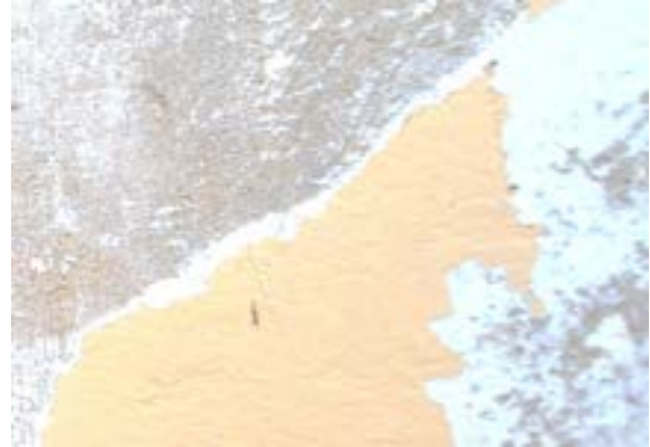
Figure 2. 198. Gypsum topcoat, smooth and hard but vulnerable to water damage. Photo by author.
