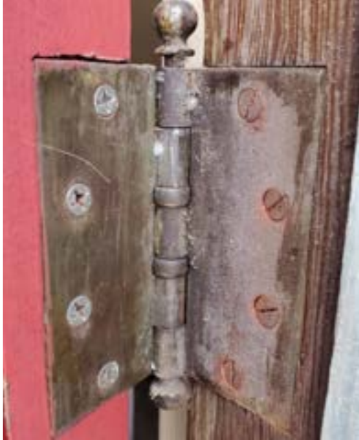
Figure 2.161. Hinges appear to be historic. Note the absence of any older hinge mortises. The door is likely not original. Note Phillips head screws versus jamb side. Photo by author.
