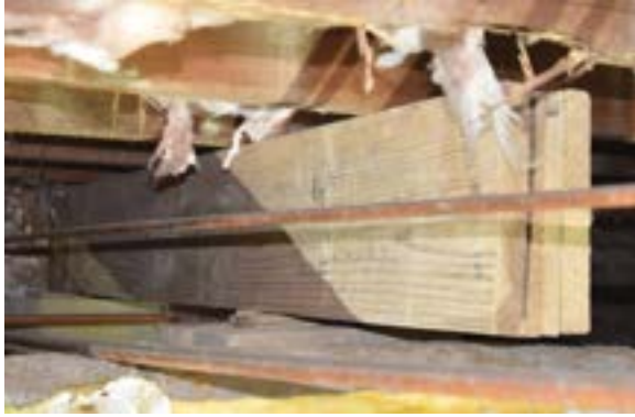
Figure 2.15. Evidence of repairs. A multiply wood beam captures weight of floor but not exterior wall. Photo by author.
