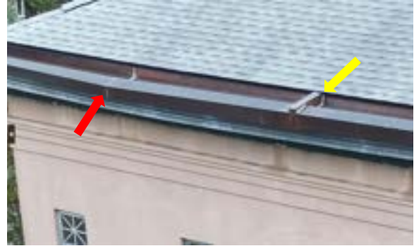
Figure 2.83. Box gutter on addition's western side. Note sag (red) and disengaged retention bracket (yellow). Photo by author.
