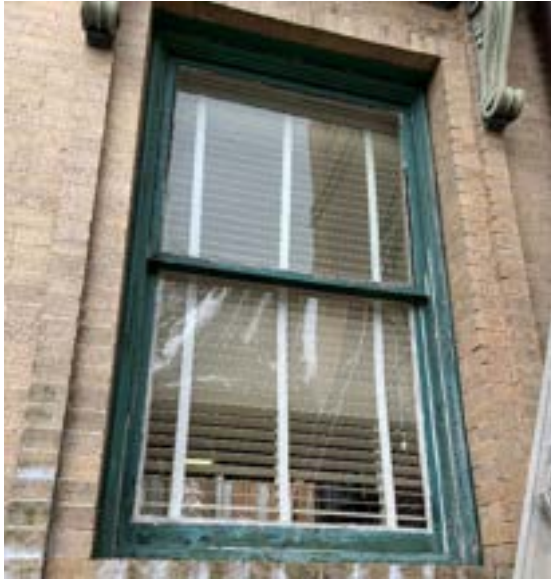
Figure 2.117. There are thirty-two one-over-one, double sash windows in the historic building. Photo by author.
