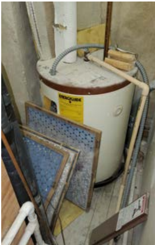
Figure 2.304. Electric powered water heater. Photo by author.
