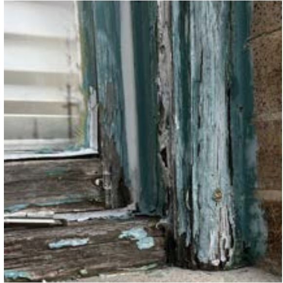
Figure 2.125. Exterior wood frames with molding. The condition of these frames and molding vary greatly around building. Photo by author.
