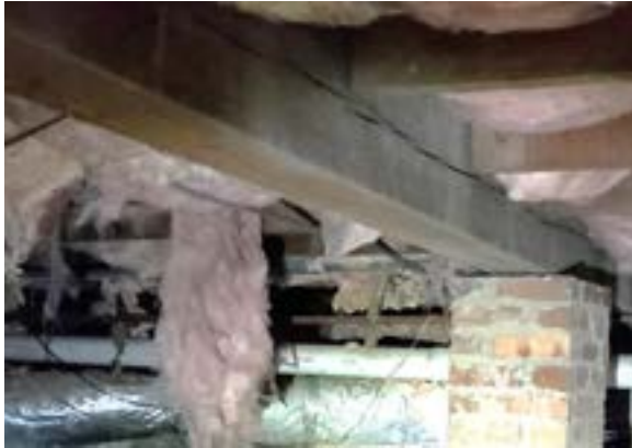
Figure 2.34. One of a pair of 6" x 8" girders in crawlspace. No lap or scarf joints observed in these 26' timbers. Photo by author.
