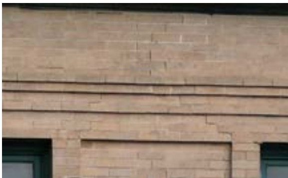
Figure 2.98. Step cracks visible in mortar on building south side. Photo by author.
