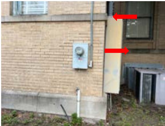
Figure 2.94. The elevation of the belt course is higher on the south side of the building. Photo by author.
