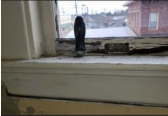
Figure 2.143. Window #206 has a heavily decayed stool. Note depth of probe. Photo by author.
