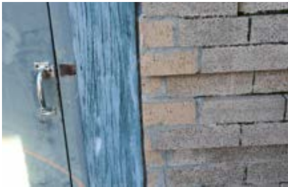
Figure 2.102. Repairs with non-matching bricks around 2nd floor fire escape door. Photo by author.
