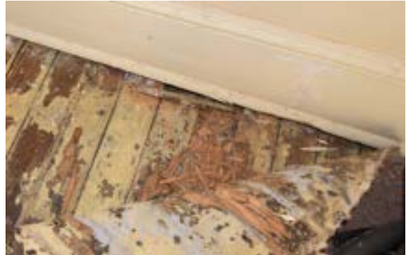
Figure 2.248. Significant material damage to 2nd floor decking in southwest corner of historic building. Photo by author.
