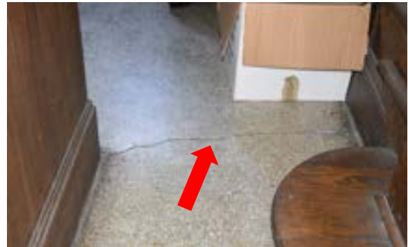
Figure 2.252. Cracks in terrazzo flooring on corresponding areas of the foyer near beginning of stairs. Photo by author.
