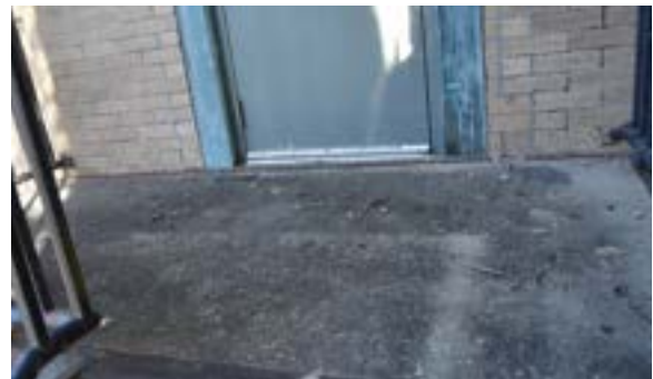
Figure 2.193. The upper fire escape platform may have been a source of water intrusion into the building in the past but tested dry during inspection. Photo by author.
