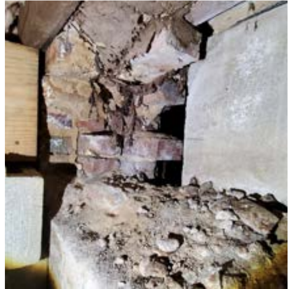
Figure 2.14. Junction of interior three wythe wall with perimeter foundation. Rear of limestone water table clearly visible on right. Photo by author.
