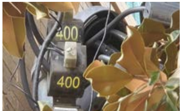
Figure 2.293. Modern service drop on southeast corner of the building. Photo by author.
