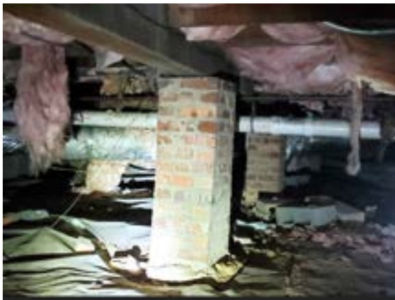
Figure 2.20. Free standing masonry columns are out of plumb, leaning to east. Photo by author.
