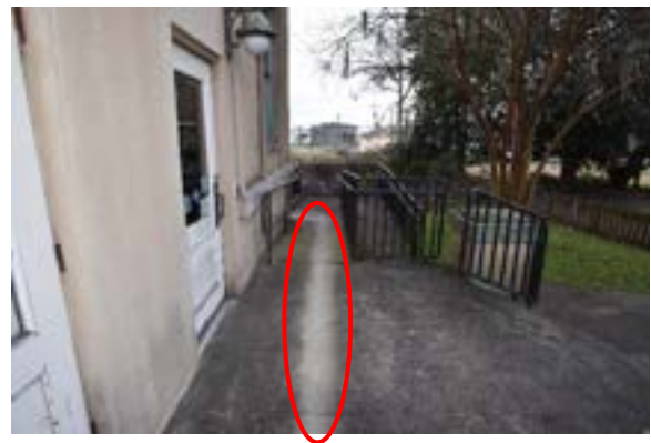
Figure 2.84. Evidence of chronic water draining onto west side concrete landing from poorly functioning box gutter above. Photo by author.
