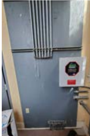
Figure 2.285. Location of old service panel. Abandoned conduit still on wall.
