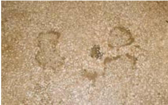
Figure 2.251. Additional patched areas in terrazzo flooring. Photo by author.
