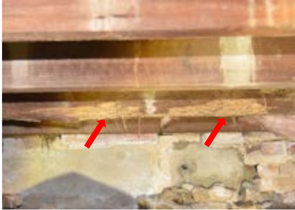
Figure 2.40. Insect damage to joists in northeast corner. Photo by author.
