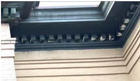
Figure 2.67. Dentil molding shows material decay and damage. Photo by author.
