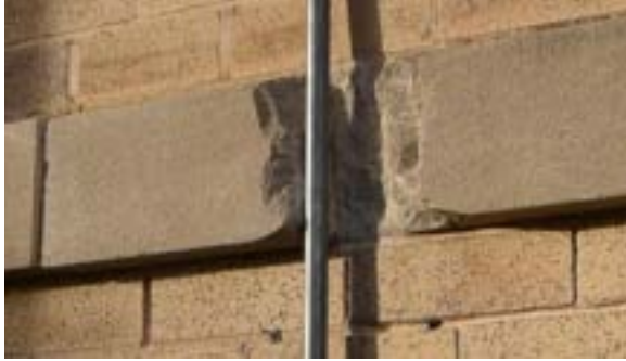
Figure 2.101. Damaged lower belt course on south side. Photo by author.
