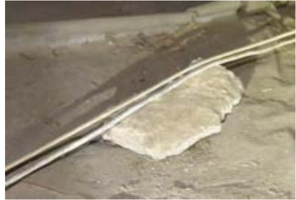
Figure 2.295. Non-code wiring in crawlspace of modern addition. Photo by author.
