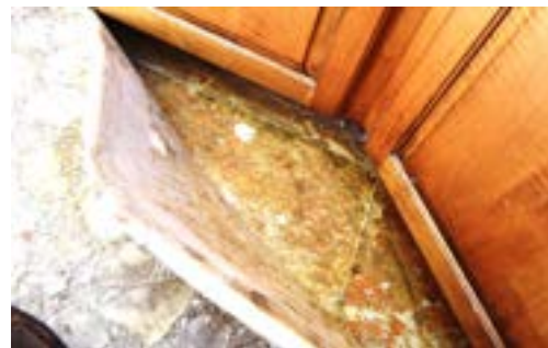
Figure 2.241. Section of kitchen floor patched with plywood. Photo by author.
