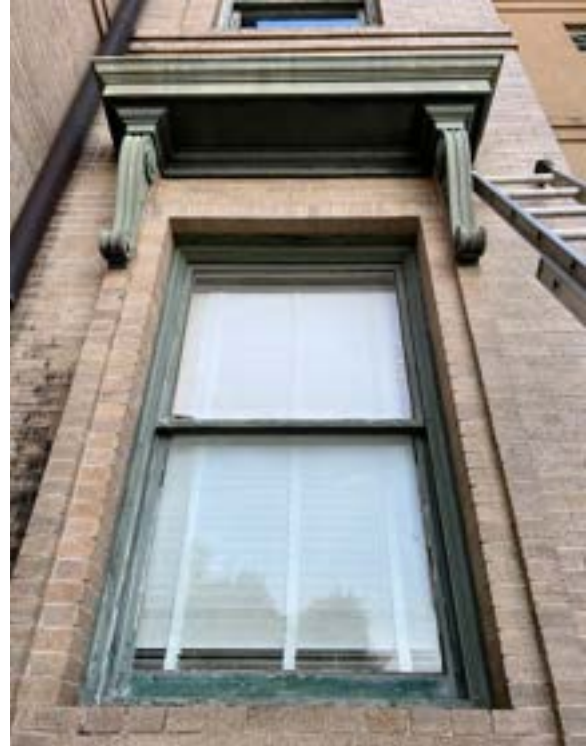
Figure 2.128. The original window hoods are located on the first-floor windows (and blind windows) along the north and east side. Photo by author.
