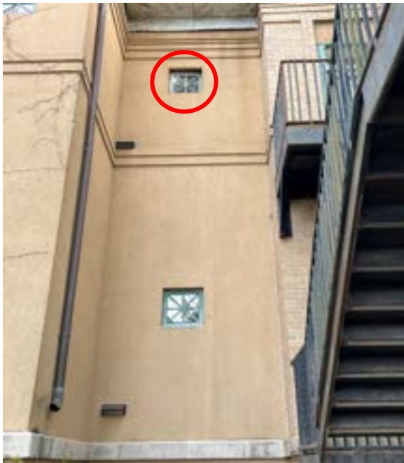
Figure 2.115. Complete weather seal failure on upper casement window on hyphen south side. Photo by author.
