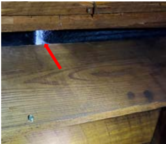
Figure 2.64. Open gap in roof system below southern end of north/south ridge line. Photo by author.
