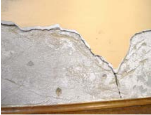
Figure 2.210. Damage to the base coat observed in places. Photo by author.
