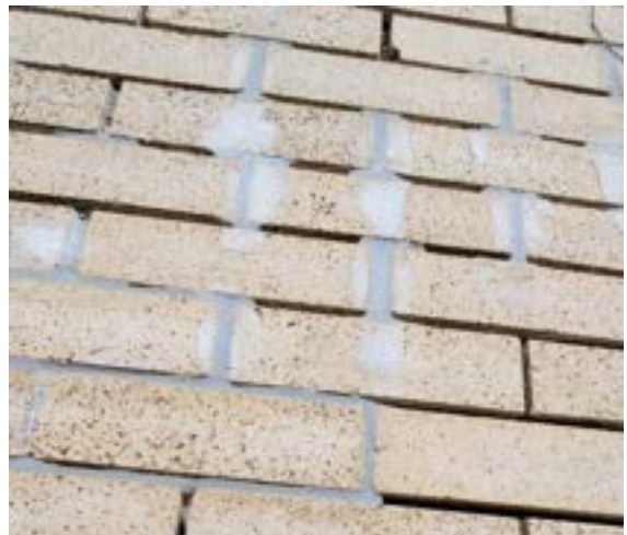
Figure 2.105. Incompatible silicone patching in building northeast corner. Photo by author.
