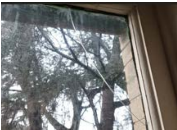
Figure 2.145. Window #204 has broken historic glass. Photo by author.
