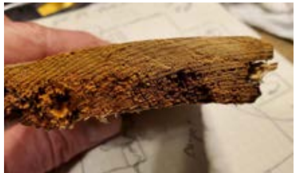
Figure 2.249. Decayed sections of 2nd floor decking. Photo by author.
