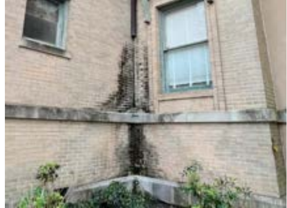
Figure 2.86. Broken downspout on historic building northwest corner resulting in significant organic growth on face brick and mortar. Photo by author.
