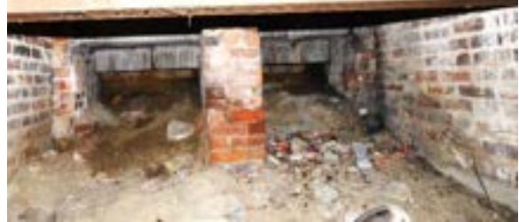
Figure 2.21. Cracks to terrazzo flooring above this section indicate possibility of foundational settling with free standing pier (center) or flanking masonry walls. Photo by author.
