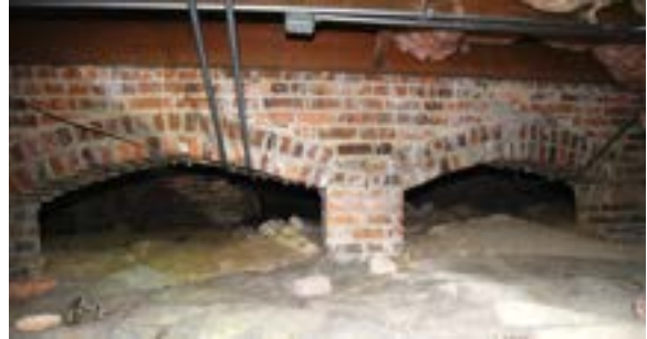
Figure 1.74. Out of sight in the crawlspace a series of beautifully constructed masonry arches line the building's northern interior wall. Photo by author.
