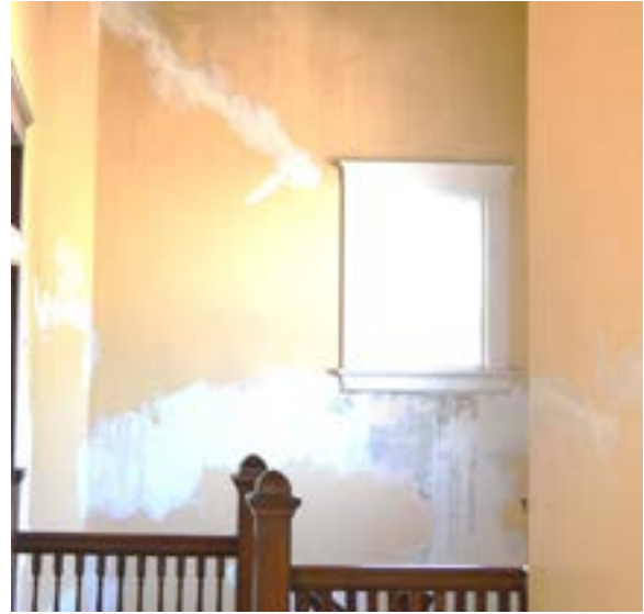
Figure 2.212. Evidence of prior repairs in western stairwell. Photo by author.
