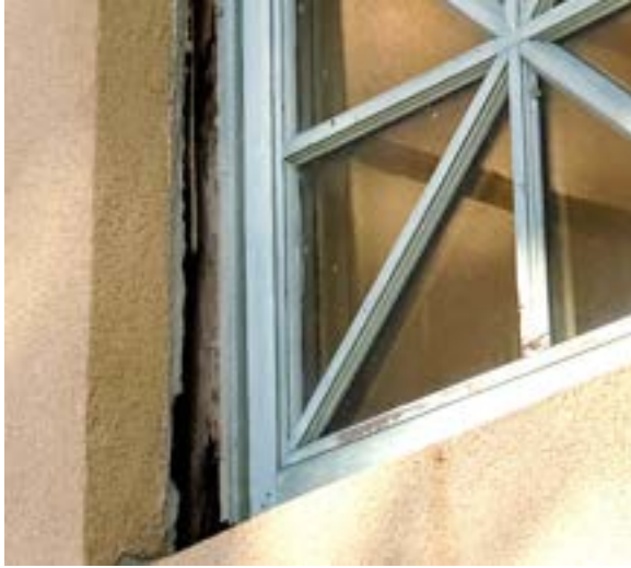
Figure 2.148. Complete EIFS separation at window frame. Photo by author.
