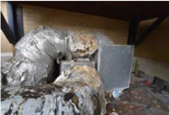
Figure 2.300. Unit B duct insulation heavily degraded. Photo by author.
