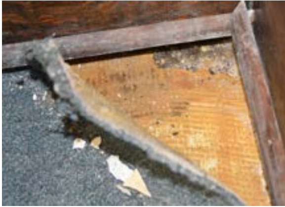
Figure 2.233. Thick layer of mastic below carpet. No padding. Photo by author.
