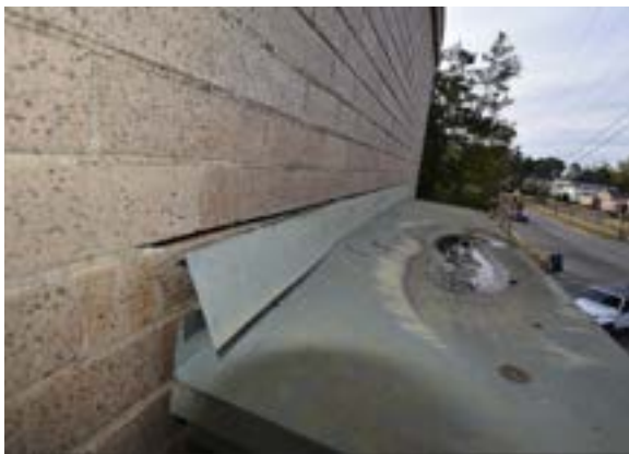
Figure 2.152. Hood H01, wall flashing separating from mortar. Photo by author.
