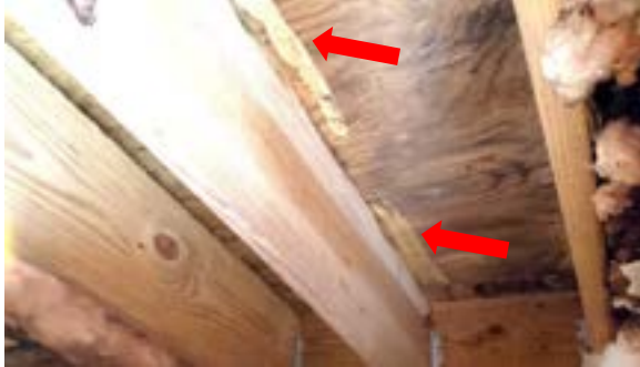
Figure 2.44. Subfloor in addition is plywood. Evidence of glue used during installation was observed (red arrows). Photo by author.
