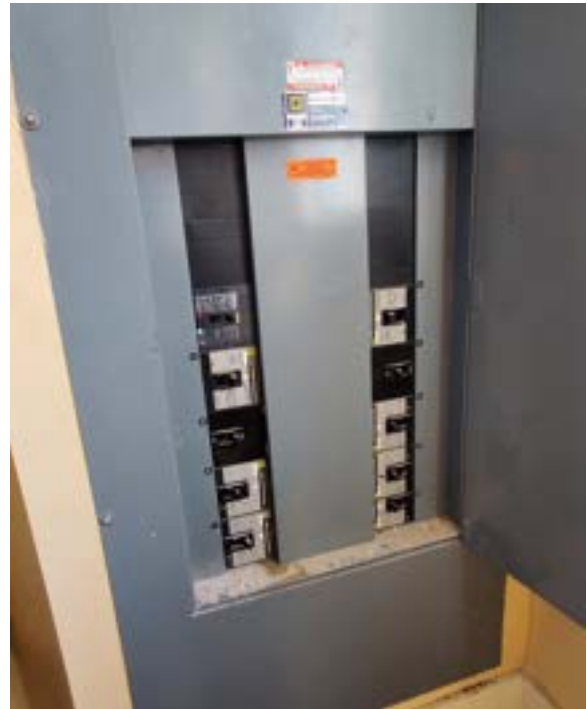
Fig. 2.288. Main panel with 400 amps of service located in second story utility rooms. Photo by author.
