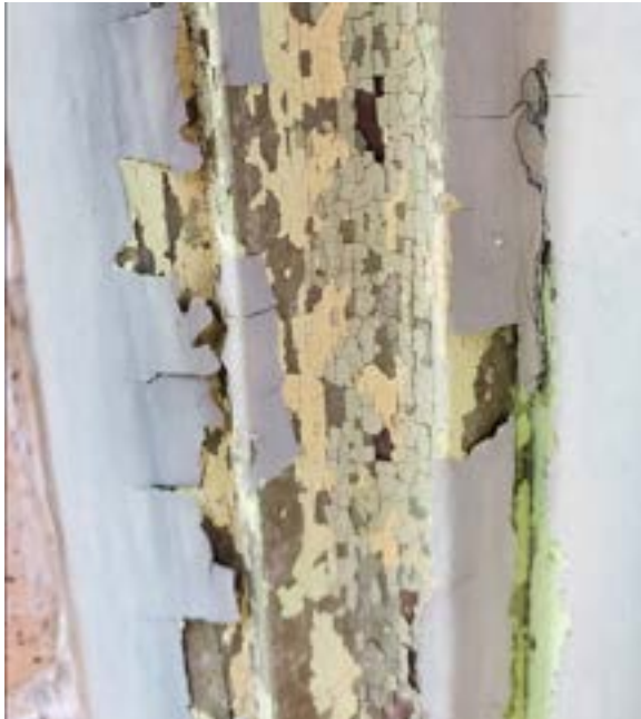
Figure 2.278. Exterior main entry door frame and trim showing a green, a yellow and an earlier shade of green. Photo by author.
