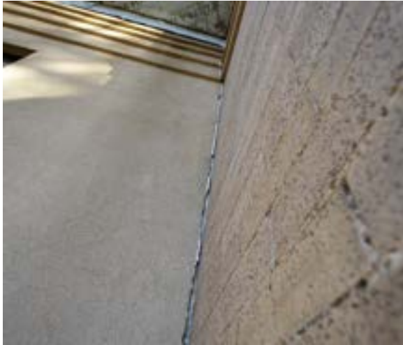
Figure 2.114. Poorly sealed vertical seam where addition joins historic building on south side. Photo by author.
