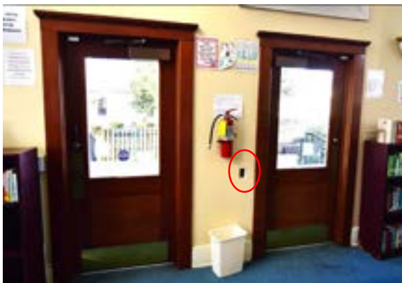
Figure 2.179. Exterior access doors on western side of addition. Note low mounted disused switch receptacle. Photo by author.
