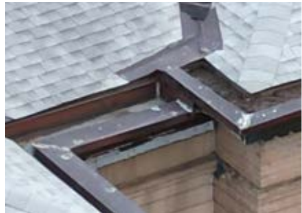
Figure 2.73. Note drop in elevation of modern addition gutter system and valley extension. Photo by author.
