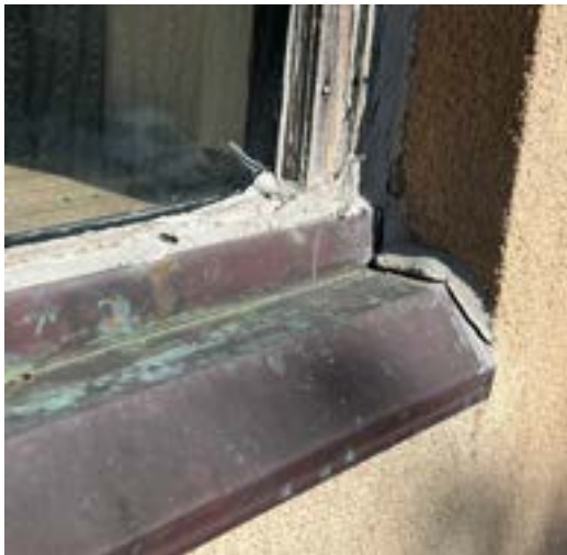
Figure 2.137. Copper sill covers appear to be a modification. Photo by author.
