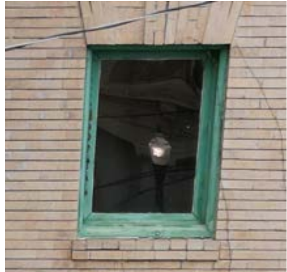
Figure 1.59. The non-historic casement window on the stairway east wall. Photo by author.
