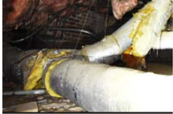
Figure 2.301. Deteriorated duct insulation and failing hangers in historic building crawlspace. Photo by author.
