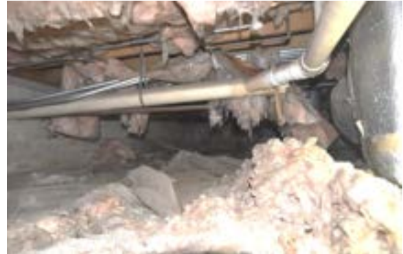
Figure 2.46. Insulation staples have rusted away causing fiberglass to fall onto crawlspace floor. Photo by author.
