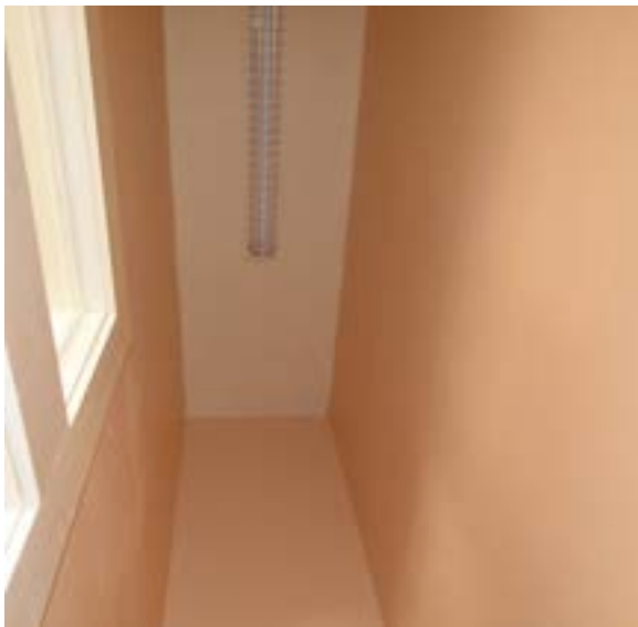
Figure 2.267. Drywall ceilings can be found throughout the historic building in areas altered by 1990s renovations. Photo by author.
