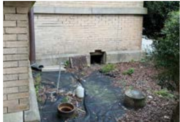
Figure 2.80. Northeast corner of building has a poor slope away from foundation causing water to pool and/or run back against foundation. Photo by author.
