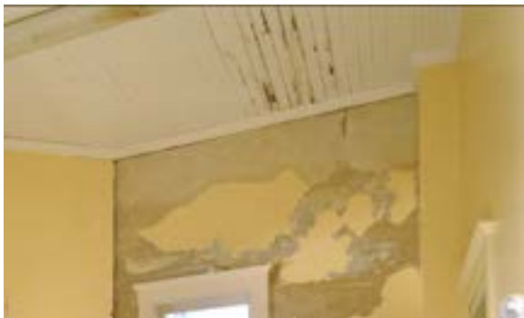
Figure 2.270. Damaged ceiling in kitchen area (west). Photo by author.
