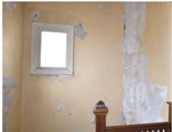
Figure 1.75. Plaster on brick finish is found throughout the building's first and second floors. Although areas are damaged, over 75% of these historic plaster walls are intact needing only cleaning. Photo by author.
