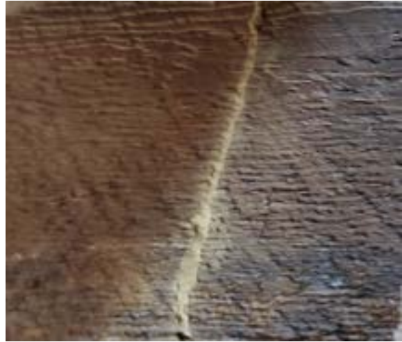
Figure 2.39. Termite trail on floor joist in crawlspace. Photo by author.
