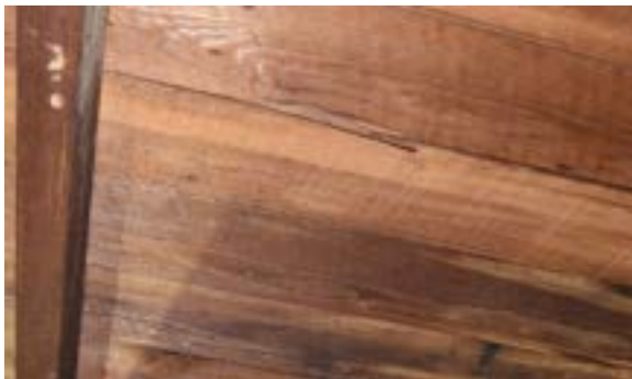
Figure 2.51. Roof decking is 1" x 5" T&G laid perpendicular to the rafters. Photo by author.
