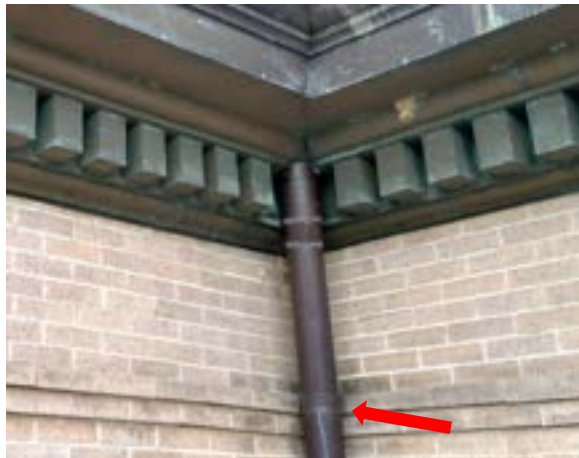
Figure 2.75. Downspouts affixed to the building exterior with copper straps. Photo by author.
