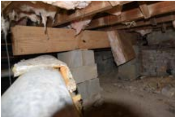
Figure 2.16. The repair beam is supported by non-mortar CMU piers. Photo by author.
