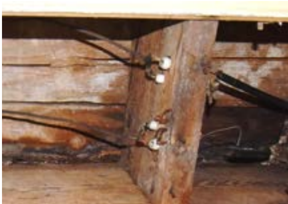
Figure 2.282. Original wiring visible in ceiling of east side foyer, beneath stairs. Photo by author.
