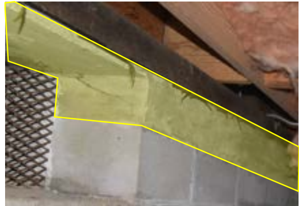
Figure 2.25. Continuous pour concrete cap (highlighted in yellow) on CMU perimeter and piers. Photo by author.
