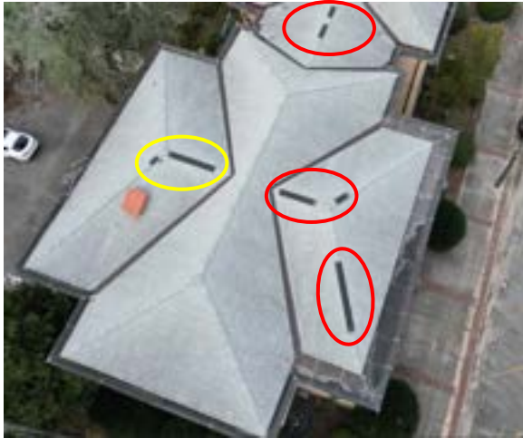
Figure 2.63. Circled areas indicate missing sections of ridge vent shingles. Photo by author.
