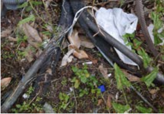
Figure 2.299. Units C & D have deteriorated insulation on coolant lines. Photo by author.
