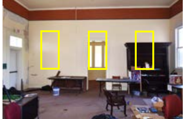
Figure 2.202. The walls on the western side of the building have drywall covering on top of the historic plaster. This is likely to cover the old window openings whose approximate locations are shown in yellow. Photo by author.
