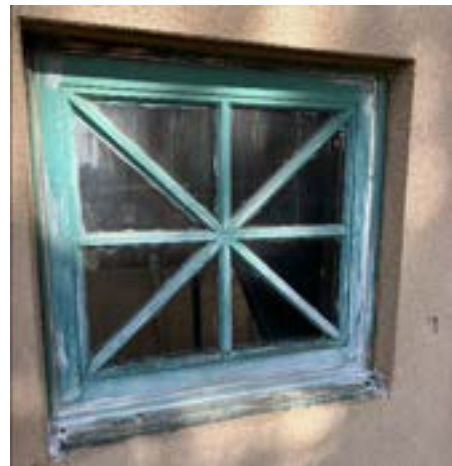
Figure 2.132. 2' x 2' starburst casements are located on all sides of the addition. Photo by author.
