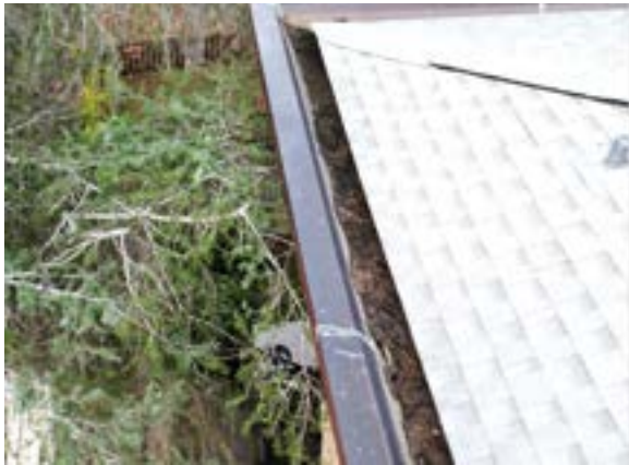
Figure 2.82. Southside historic building gutter heavily clogged with organic debris. Photo by author.
