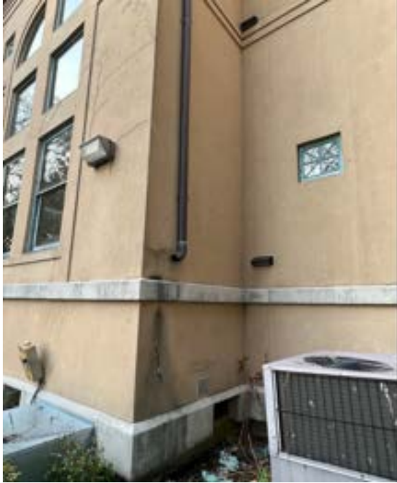
Figure 2.85. Shortened downspout on the addition's southside causing water to drain down wall. A similar situation exists with other downspouts. Photo by author.
