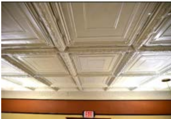
Figure 2.254. Fabricated, pressed metal ceiling is the most prevalent ceiling finish in the building. Photo by author.
