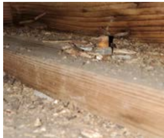
Figure 2.43. Joists fastened to 2"x 8" sill which is secured with anchor bolt in concrete cap. Photo by author.
