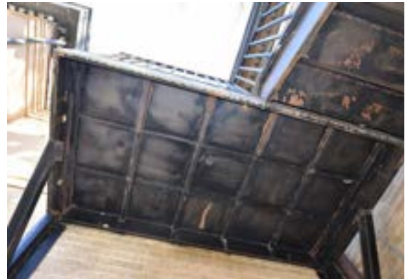
Figure 2.192. Rust evident on various fire escape surfaces. Photo by author.
