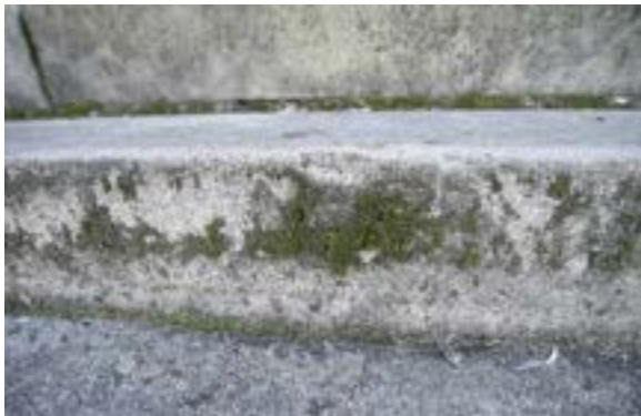
Figure 2.191. Significant organic growth on main entry stairs. Photo by author.
