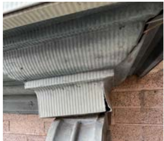
Figure 2.154. Hood H04, cornice corner and corbel have fractured. Photo by author.
