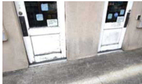
Figure 2.181. Degraded paint finishes on the addition's exterior doors. Photo by author.
