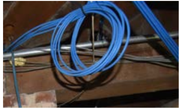
Figure 2.296. Data cable servicing first floor. Photo by author.
