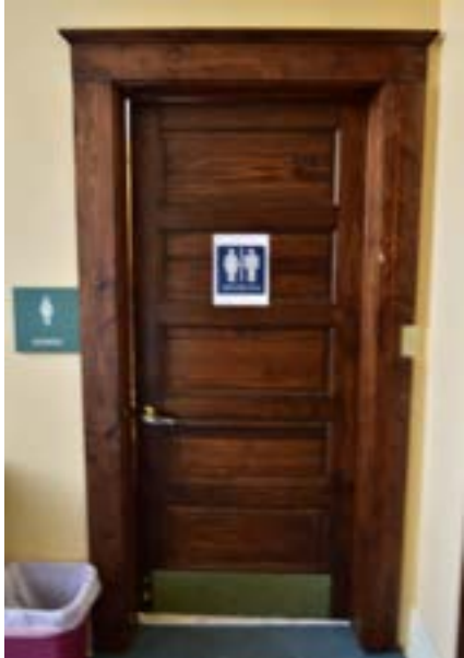
Figure 2.178. First floor restroom doors measure 36" across. Photo by author.
