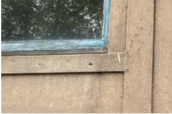
Figure 2.110. In addition to punctures to the veneer, window openings have also been noted to fail. Photo by author.
