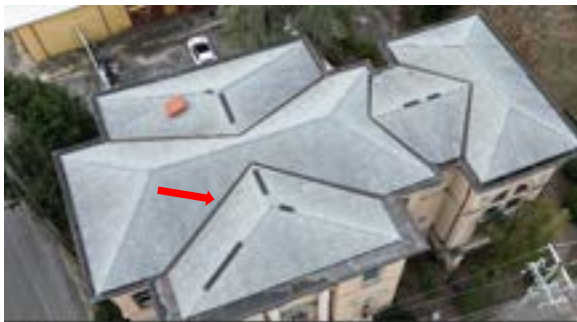
Figure 2.71. Eight copper lined valleys (one highlighted in red) drain water to the gutters. Photo by author.
