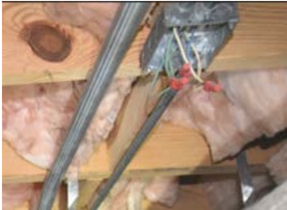
Figure 2.294. Numerous uncovered junction boxes were found throughout the building. Photo by author.
