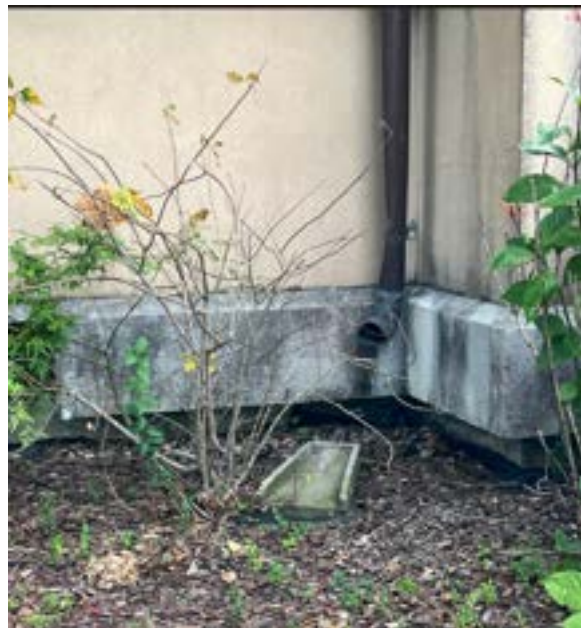
Figure 2.77. Downspouts are intended to terminate at an elbow drain near grade, but most are broken or disconnected. Photo by author.
