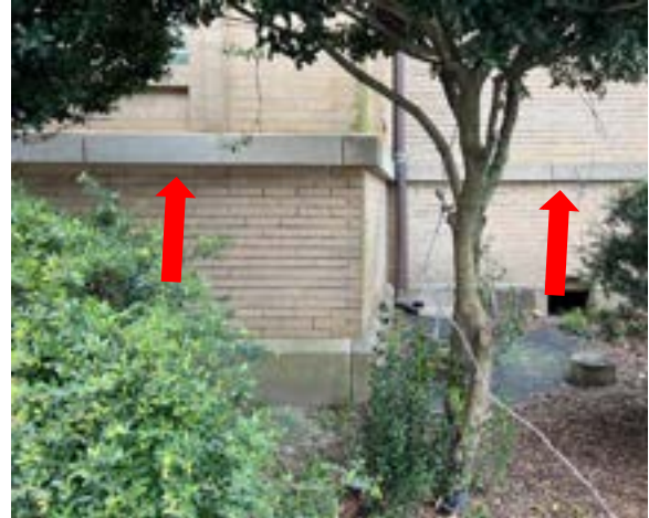
Figure 2.91. The historic building has one limestone belt course (red arrows). Photo by author.
