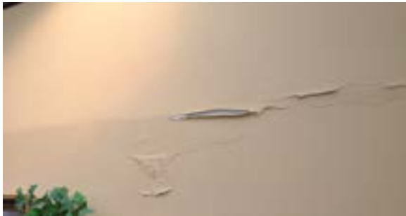
Figure 2.214. Drywall damage on east wall of modern addition. Photo by author.
