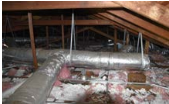
Figure 2.302. Ducting and insulation in attic in good condition. Photo by author.
