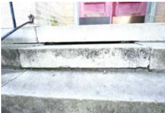
Figure 2.187. Settling evident to granite block on upper tread. Photo by author.
