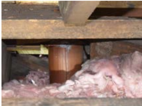
Figure 2.74. Copper downspouts cut through the cornice assembly inside the box gutter. Photo by author.
