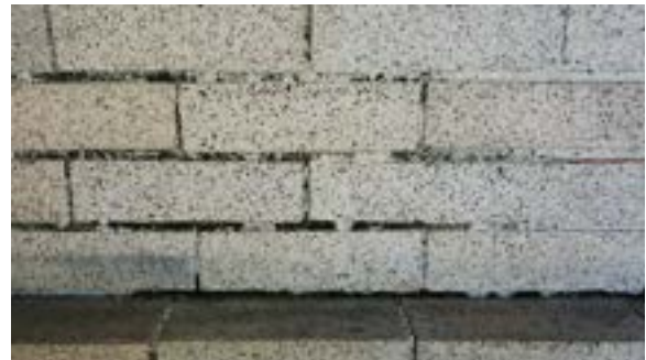
Figure 2.100. Organic growth on mortar widespread in low sunlight areas on all sides of the historic building. Photo by author.
