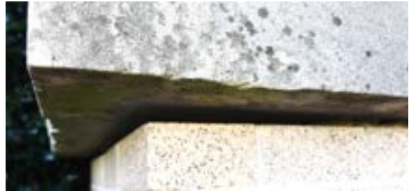
Figure 2.104. Significant mortar recession beneath entire length of limestone belt course on north side. Photo by author.
