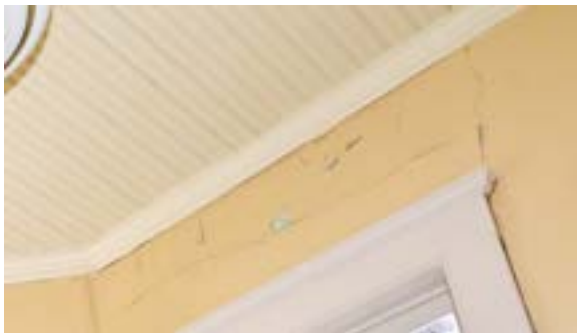
Figure 2.211. Two instances of plaster damage due to load shifting or settling. Photo by author.
