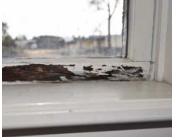
Figure 2.146. Window #119 has extensive material damage on modern window sash. Photo by author.
