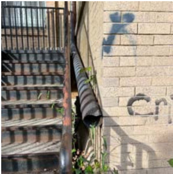
Figure 2.79. Southside historic building downspout terminates well above grade. Photo by author.
