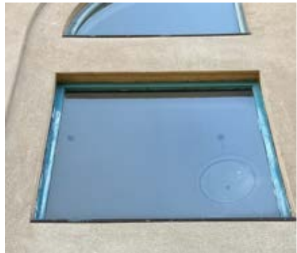
Figure 2.135. No formal exterior casing on addition windows. Photo by author.
