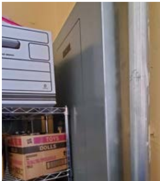
Figure 2.291. Panel "A" inaccessible due to bookshelf. Photo by author.
