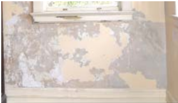
Figure 2.197. Base coat integrity is good in damaged areas. Photo by author.
