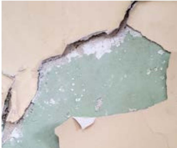
Figure 2.275. Damaged wall section showing possible paint chronology. Photo by author.
