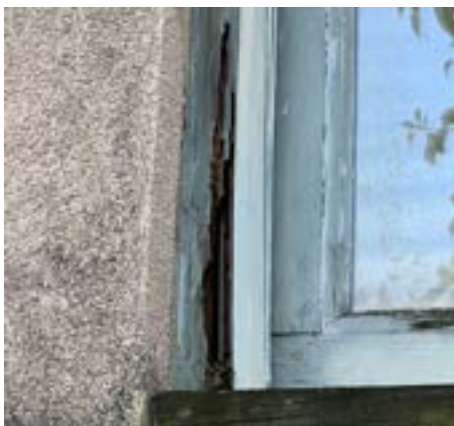
Figure 2.150. Fully decayed window frame. Photo by author.
