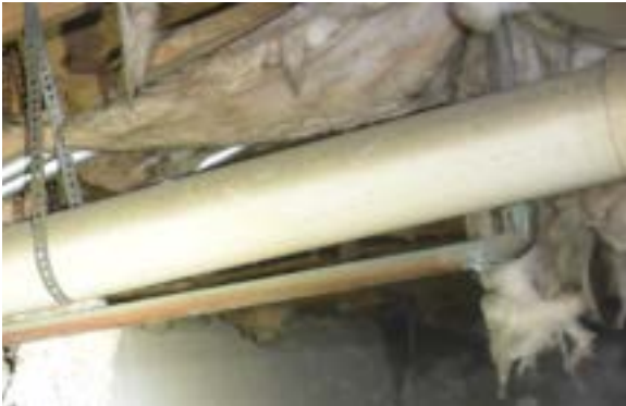
Figure 2.308. PVC waste and copper supply lines observed in modern addition crawlspace. Photo by author.
