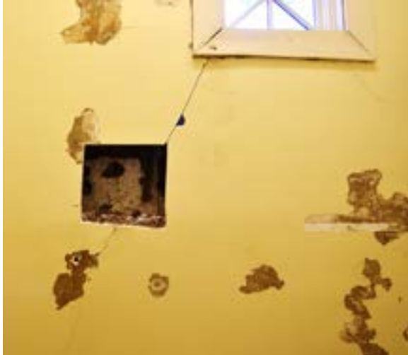
Figure 2.213. The damaged wall finish in 2nd floor southside restroom. Photo by author.
