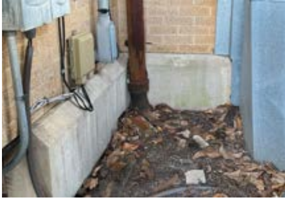
Figure 2.78. Southeast corner historic building downspout drains into cast iron city waste line. Photo by author.
