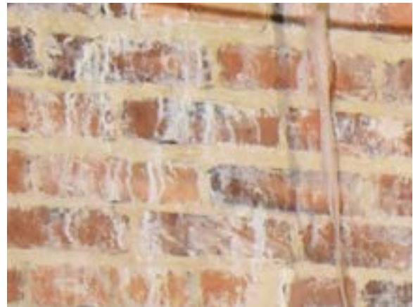
Figure 2.18. Evidence of efflorescence at various locations on perimeter wall. Photo by author.
