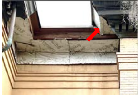
Figure 2.65. Missing section of hyphen roof cornice and southwest corner of historic building. Photo by author.
