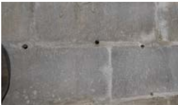
Figure 2.24. Weeps holes in mortar joint on inside of the addition foundation walls. Photo by author.
