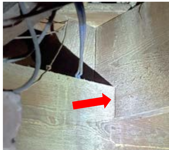
Figure 2.36. Floor joists notched on carrying beam. No evidence observed of checking (cracking) at notch which is common. Photo by author.
