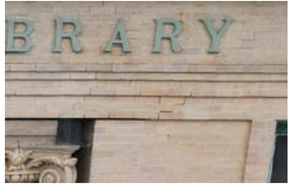
Figure 2.99. Step cracks on either side of building name north side. Photo by author.
