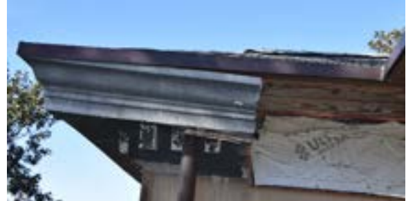
Figure 2.68. Missing section of cornice on southside of addition. Photo by author.
