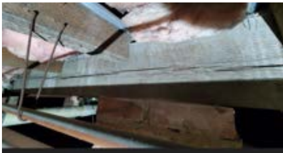
Figure 2.38. Some checking observed in long carrying beams. Photo by author.
