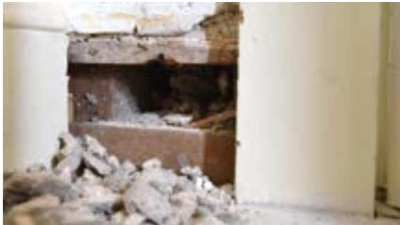
Figure 2.175. Historic framing located inside the non-historic wall on second floor. Photo by author.
