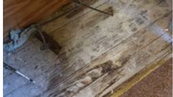
Figure 2.239. Unfinished wood floor section in 2nd story utility closet. Photo by author.
