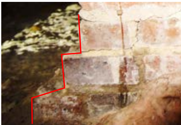
Figure 2.5. Exposed corbelled spread footer (outlined in red) below engaged piers. Photo by author.
