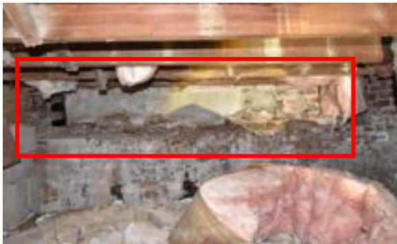
Figure 2.13. Demolished section of perimeter wall in northeast corner measures 8' x 16". Photo by author.
