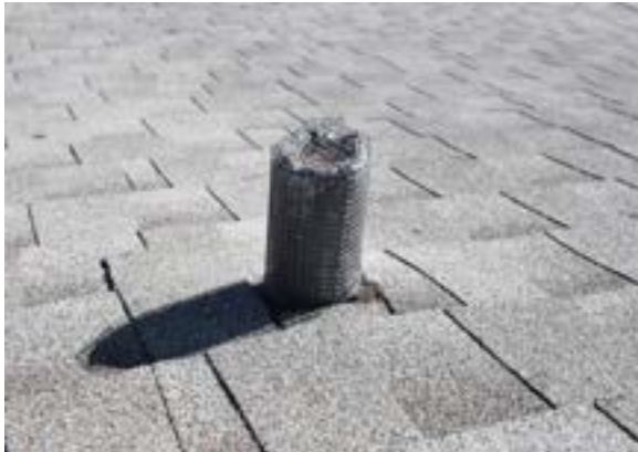
Figure 2.70. One of the six plumbing vent penetrations in roof. Photo by author.
