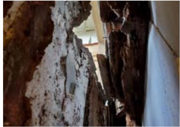
Figure 2.116. Full material failure inside the load bearing wall behind the casement window, hyphen south side. Photo by author.
